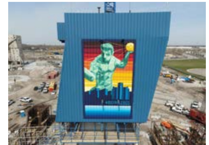
A mural depicting the Spirit of Detroit at the US bridge site
